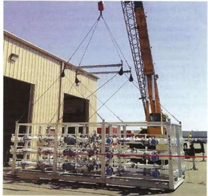
FIG. 2. Railcar loading skid with strainers, flowmeters, pressure regulators and prover connections for use in bulk liquid terminal operations. Photo courtesy of ShureLine Construction.
