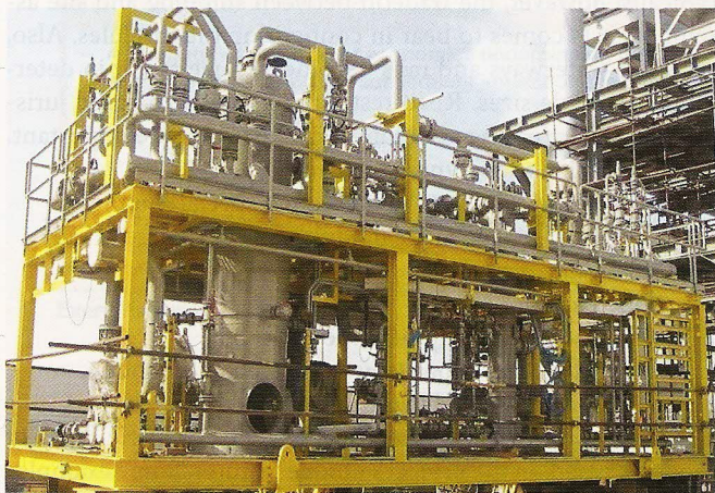
FIG. 1. Flue gas conditioning module. Photo courtesy of Descon Engineering.
