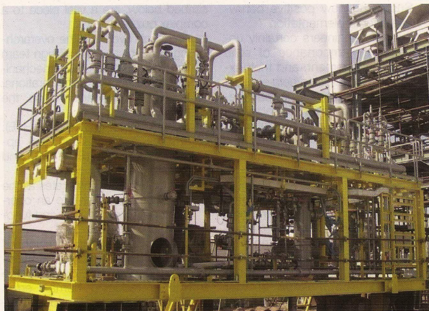
FIGURE 1. This photo shows a fluegas-conditioning module, which is part of a large process plant that was fully fabricated in a local shop in the Middle East to achieve the desired schedule
