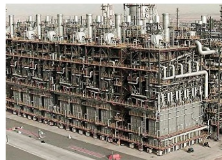
FIG. 3. Large ethylene furnace with modular sections.
